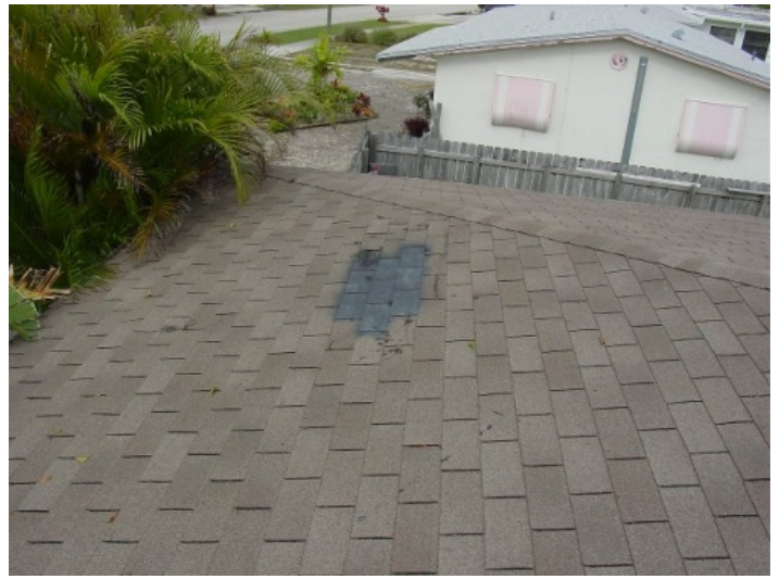
Hip roof - some shingle replaced on the front left side
